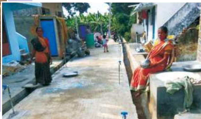
Piped water supply in Garividi cluster, Vizianagaram, Andhra Pradesh
