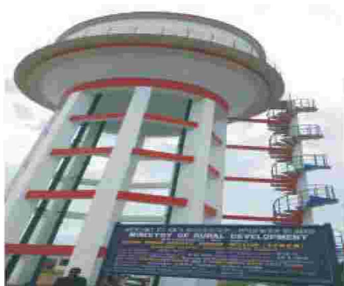
Overhead Water Tank in Khangabok cluster, Thoubal District, Manipur
