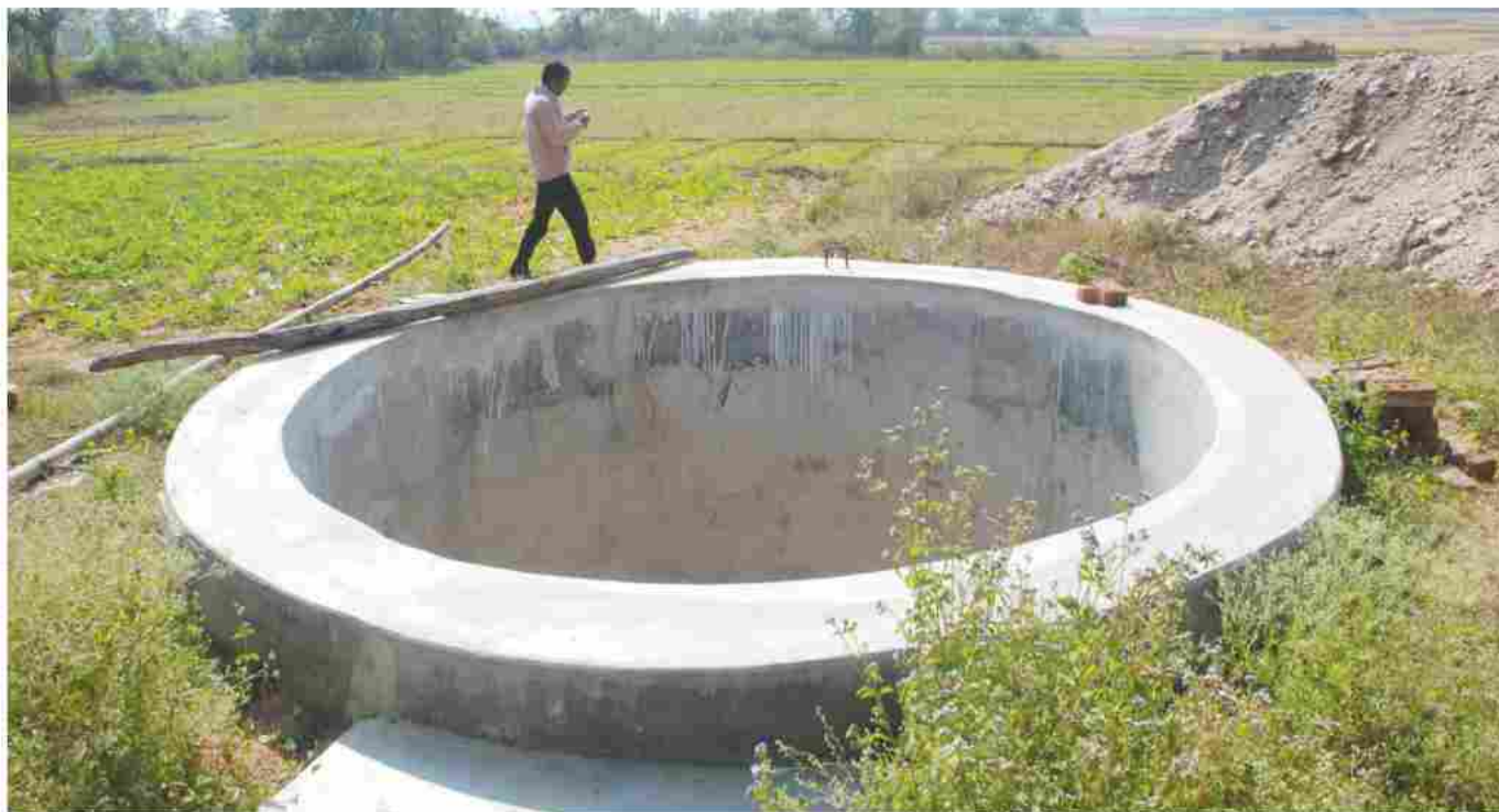
Irrigation Well - MGNREGA Vill. Dharmu, G.P. Hadari, Block Ichak, Distt. Hazaribagh, Jharkhand
